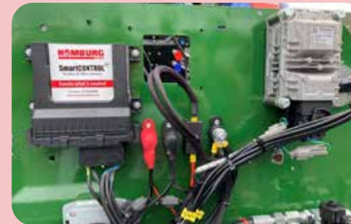
▲ SmartCONTROL & USC modules
